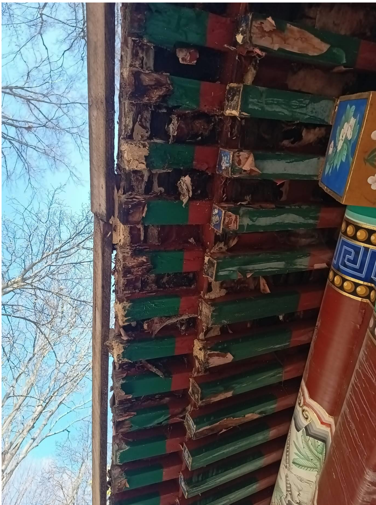
Photo 11. Fibroporia vaillantii on the rafters of the Chinese Pavilion (photo: Marta Wrzosek)
